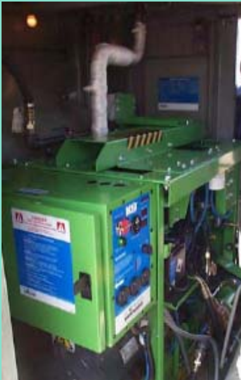
Auxiliary Power Unit
